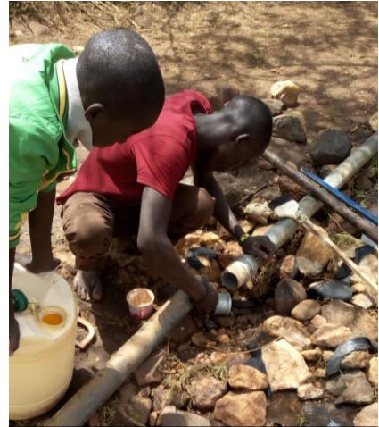
A plumber working on a leaking pipe at the Mission Station. As soon as the water charges are instituted, this water project will be able to sustain its servicing and maintenance and also earn income to the Station.
